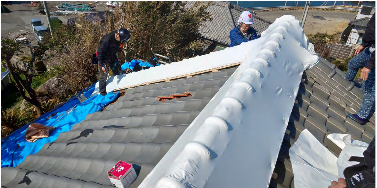
Shrink wrap roofing material was used to repair roofs for the near-term. Photo: Osekkaï
